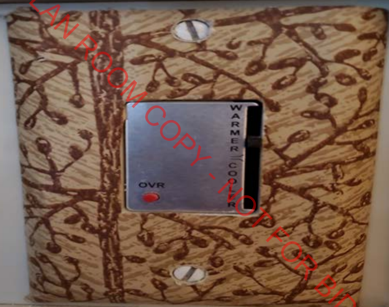
AAON Unit Thermostats (Unit #2 & #7)
