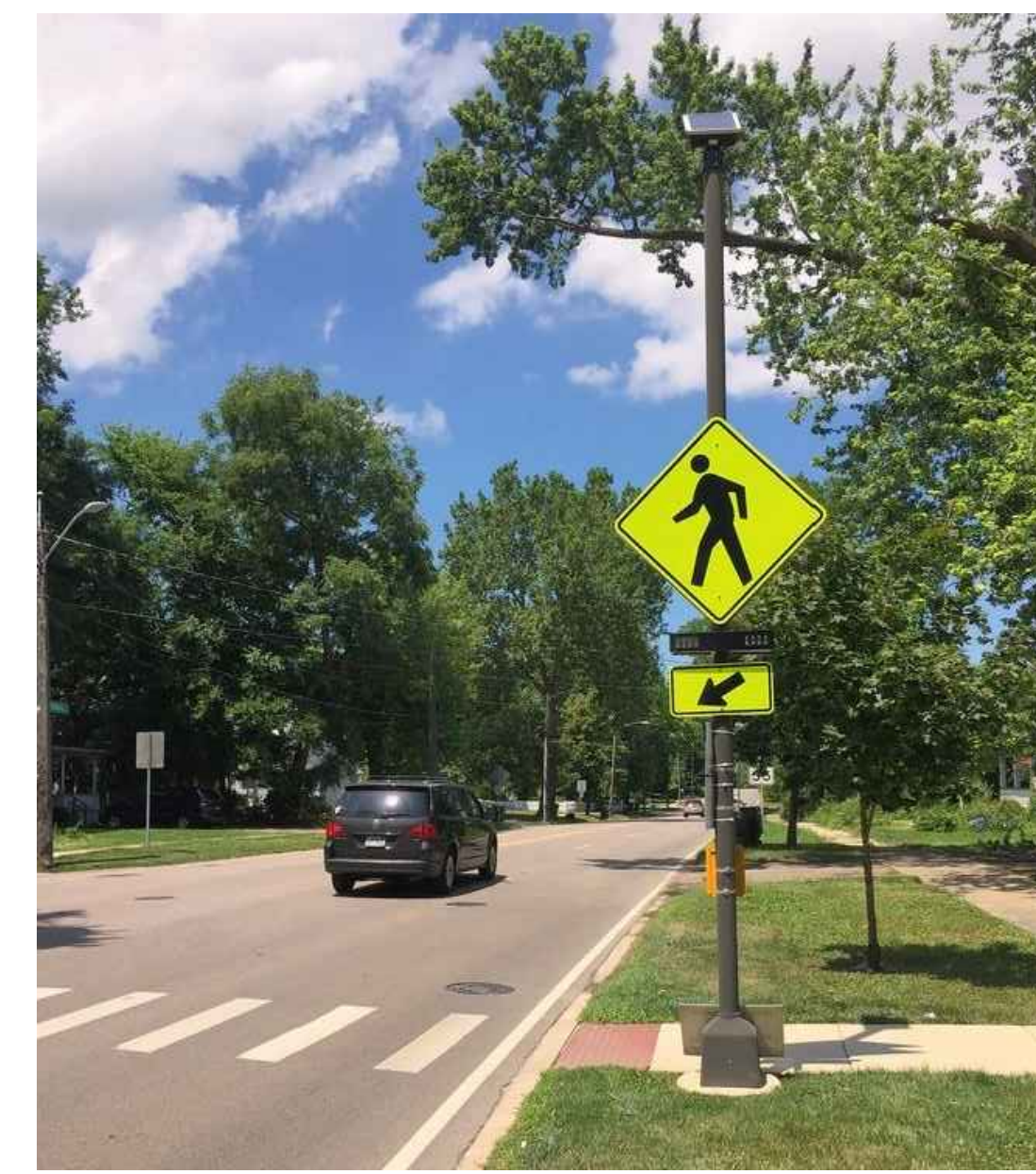
Trail Crossing with Solar Safety Beacon Lights / Signage
